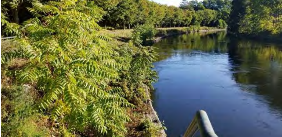
Polygon No.: 79 Photo No.: 79 Date: 9/27/2019 Direction Photo Taken: Northeasterly Description: Tree of heaven trees and vines are growing on top of the canal wall and within approximately 3 feet of the canal wall.
