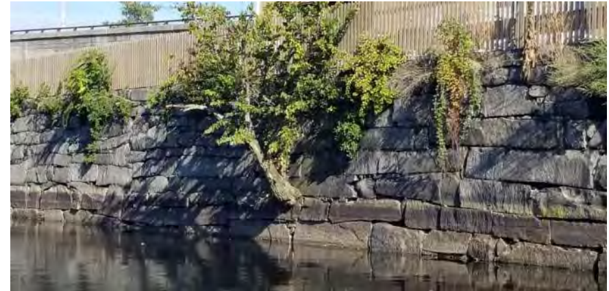
Vegetation Point No.: VP-16 Photo No.: VP-19 Date: 9/26/2019 Direction Photo Taken: Northerly Description: A small clump of mulberry are growing out of the canal wall.
