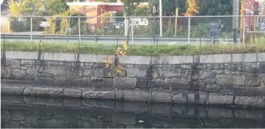
Vegetation Point No.: VP-10 Photo No.: VP-13 Date: 9/26/2019 Direction Photo Taken: Southerly Description: A small maple is growing out of the canal wall, near the top of the wall.
