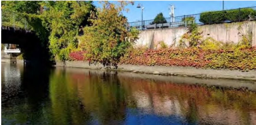
Polygon No.: 56 Photo No.: 56 Date: 9/26/2019 Direction Photo Taken: Southwesterly Description: Most of the canal wall is made of concrete with riprap placed at the toe of the wall. The vegetation growing on the canal wall consists of tree of heaven, box elder, and vines, such as Boston ivy.
