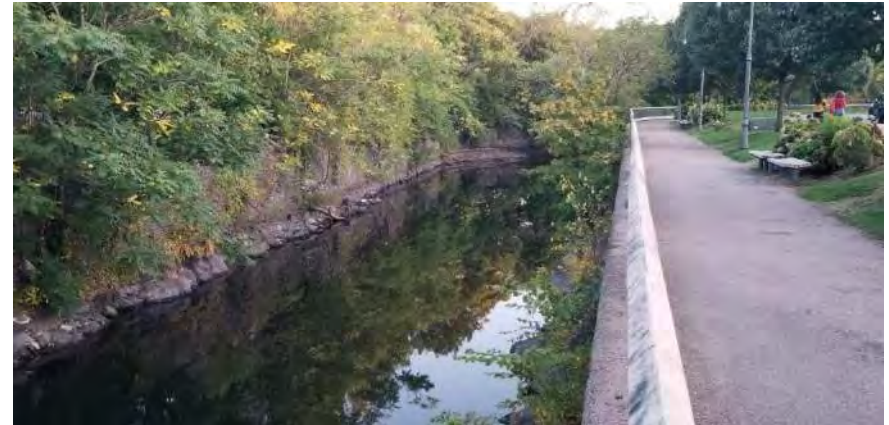
Polygon No.: 41 Photo No.: 41b Date: 9/25/2019 Direction Photo Taken: Southeasterly Description: Portions of the canal wall at bridge crossings on each side of the canal are concrete and brick. The highest density of vegetation in the polygon consists of locust, tree of heaven, box elder, maples and scattered shrubs, some with approximately 6 to 14 inches diameter at breast height.
