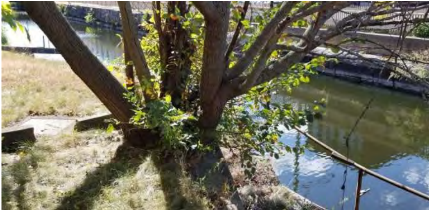
Polygon No.: 13 Photo No.: 13 Date: 9/25/2019 Direction Photo Taken: Southerly Description: There is one elm tree and one mulberry growing out of concrete portion of the canal wall.
