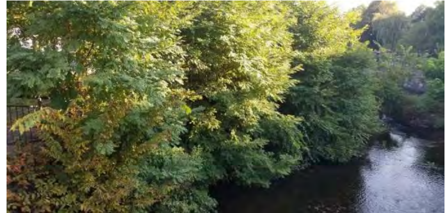
Polygon No.: 47 Photo No.: 47 Date: 9/26/2019 Direction Photo Taken: Northeasterly Description: The vegetation growing on the canal wall includes large locust trees and ragweed.
