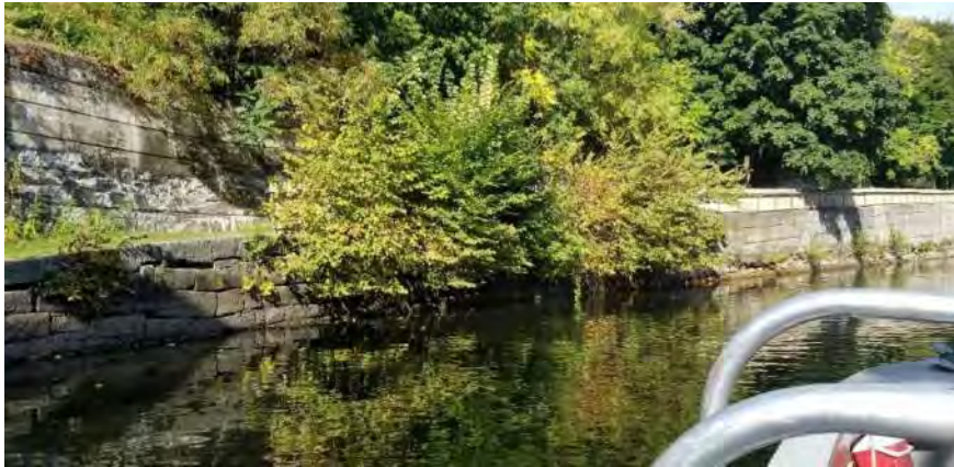
Polygon No.: 69 Photo No.: 69 Date: 9/26/2019 Direction Photo Taken: Northwesterly Description: The trees growing out of canal wall include tree of heaven and elms at approximately 10 feet tall.
