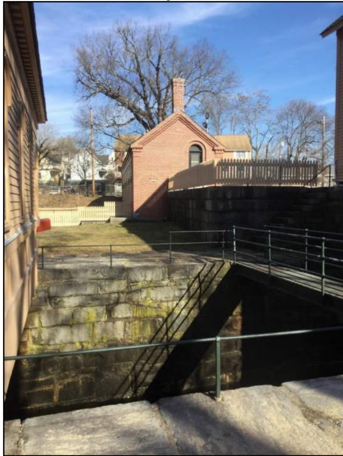
Figure E.7-32. Guard Lock and Gates Facility.
