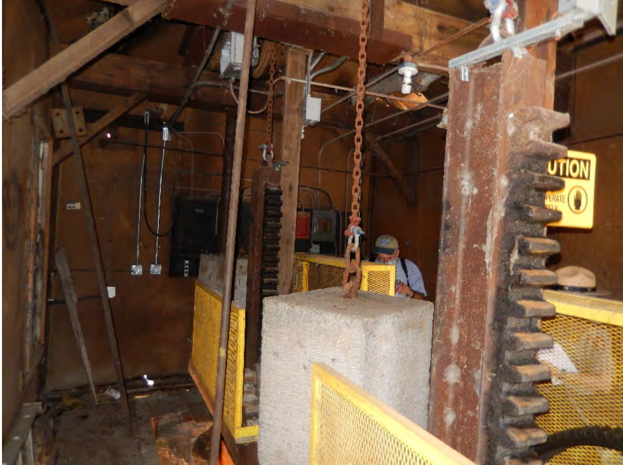
Figure 5-1. Hamilton Wasteway Gate House, rack-and-pinion hoisting mechanism.
