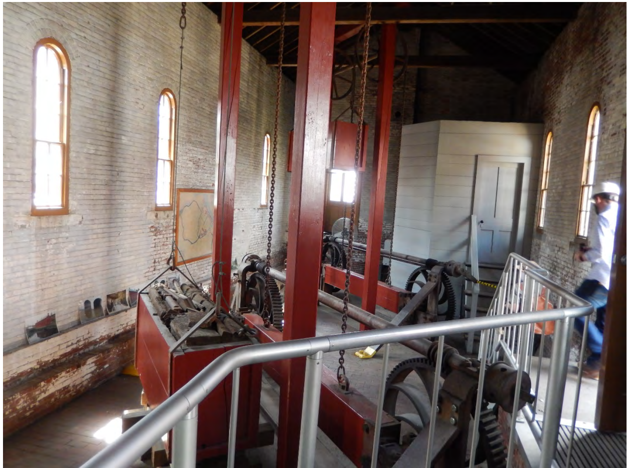
Figure 6-1. Moody Street Gate House, gate hoisting mechanisms.
