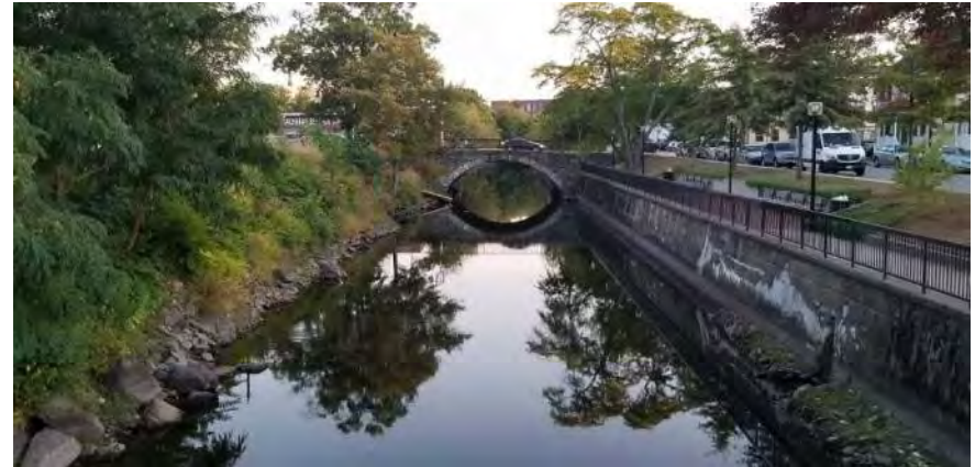
Photo Location No.: P-3 Date: 9/25/2019 Direction Photo Taken: Southwesterly Description: Vegetation is growing on the riprap shoreline located on the eastern side of the canal (left side of the photograph). The western side of the canal wall (right side of the photograph) is concrete with little to no vegetation present.
