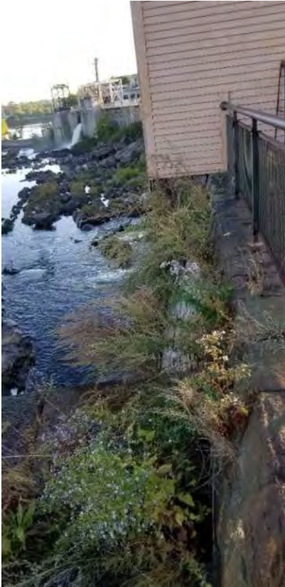
Polygon No.: 74 Photo No.: 74 Date: 9/27/2019 Direction: Northeasterly Description: Ragweed is growing out of the canal wall located beneath the building.
