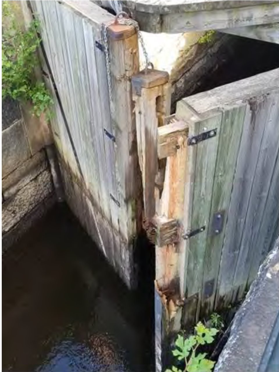
Photo 5-3. Damage to the Northern Canal Lock Timber Gate.
