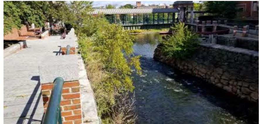
Polygon No.: 7 Photo No.: 7a Date: 9/25/2019 Direction Photo Taken: Easterly Description: Several large woody trees including river birch, tree of heaven, and silver maple, all approximately 2 to 5 inches diameter at breast height are growing out of the canal wall.
