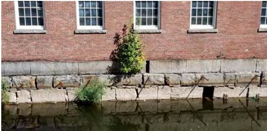
Vegetation Point No.: VP-1 Photo No.: VP-4 Date: 9/25/2019 Direction Photo Taken: Northeasterly Description: Vegetation includes a single shrub growing out of the canal wall below the brick building and sparse herbaceous species.
