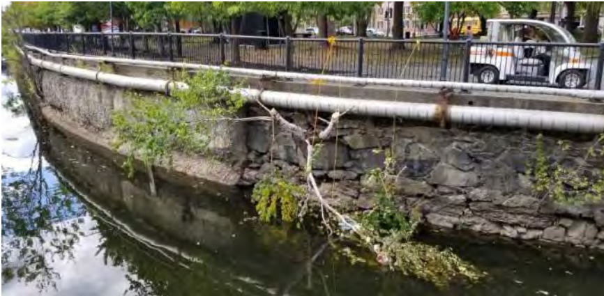
Polygon No.: 90 Photo No.: CV_Poly10a Date: 9/25/2019 Direction Photo Taken: Southwesterly Description: The vegetation growing out of canal wall is a 3-trunked tree of heaven tree at approximately 4 inches diameter at breast height. A recently cut birch tree tied with rope was also observed along the canal wall.
