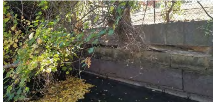
Polygon No.: 57 Photo No.: 57 Date: 9/26/2019 Direction Photo Taken: Easterly Description: Vegetation growing out of the canal wall includes ash trees at approximately 6 to 8 inches diameter at breast height.
