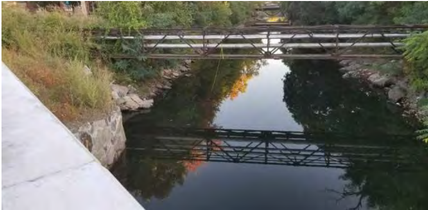
Photo Location No.: P-2 Date: 9/25/2019 Direction Photo Taken: Southwesterly Description: Vegetation is growing on the riprap shoreline along both sides of the canal.
