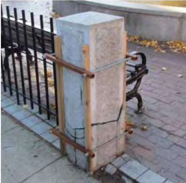
A cracked granite post and temporary wooden support structure in the Mack plaza. (DCR)
