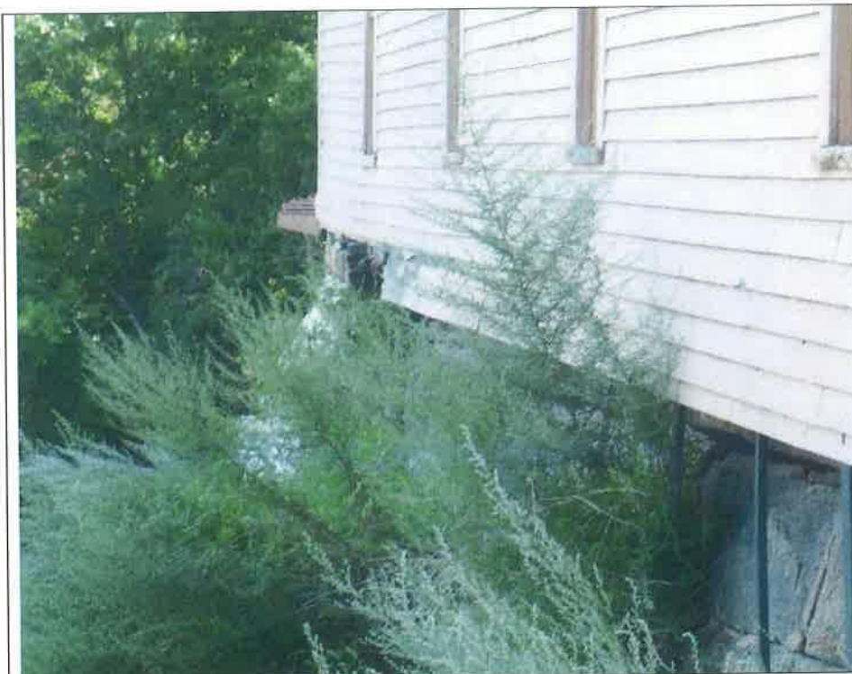
Photograph 3 – Deteriorated / missing sill and missing siding boards at eastern end of north wall; entire building has settled in this area, as evidenced by the downward curvature of the siding boards under the left-most window.
