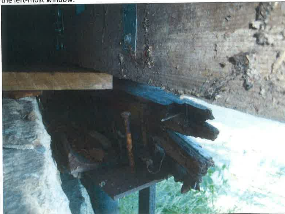
Photograph 4 – Deteriorated / missing sill under eastern edge of north wall; note large gap between dam and wall.
