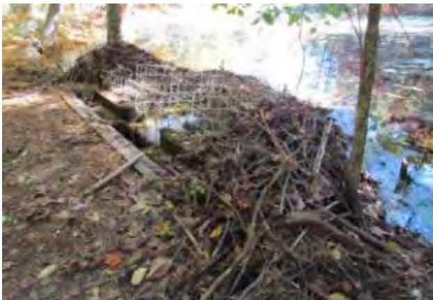
A culvert at the intersection of Woodchuck Trail and Garrison Loop. (DCR)
