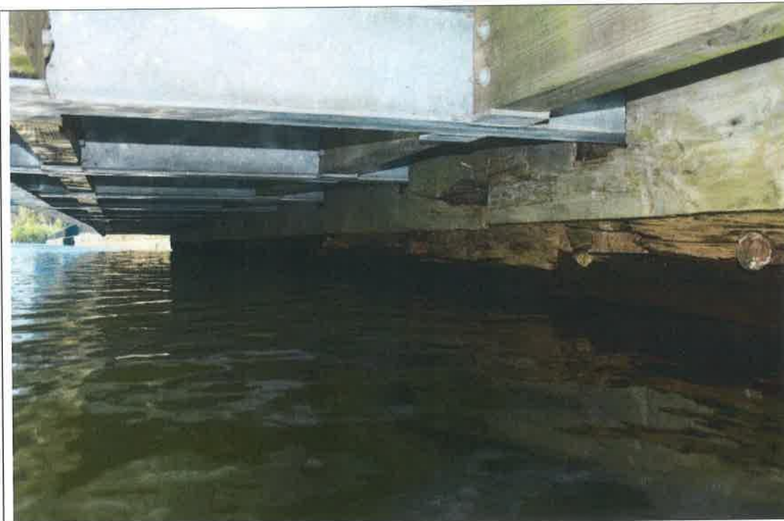
Photograph 7 – Underside of walkway along south side of gatehouse; the deteriorated sill that is now partially submerged in water is visible in Photographs 5 and 6.
