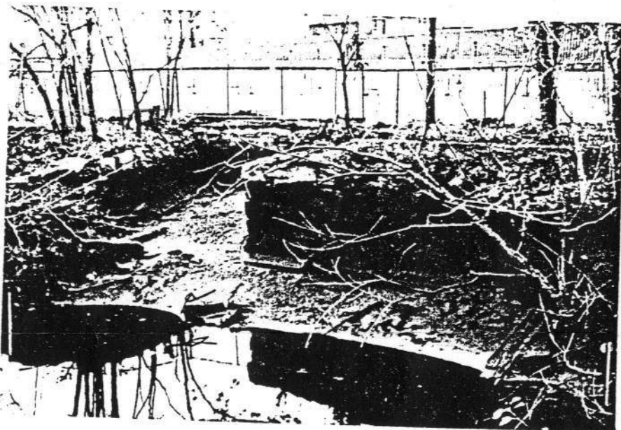
Detail of the Machine Shop head race off the Merrimack Canal, shown when the canal was drained. Photo taken in October 1979.
