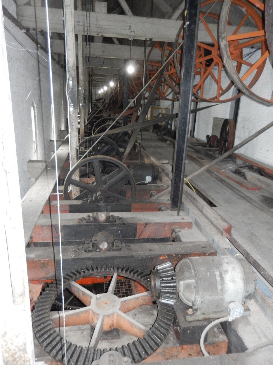
Figure 5-5. Pawtucket Gate House, belt-and-line shaft system with electric motor drive in foreground.
