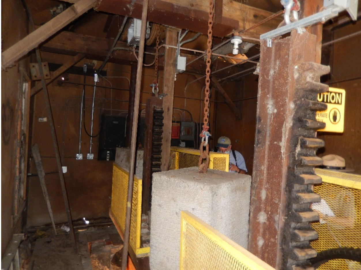
Figure 5-1. Hamilton Wasteway Gate House, rack-and-pinion hoisting mechanism.
