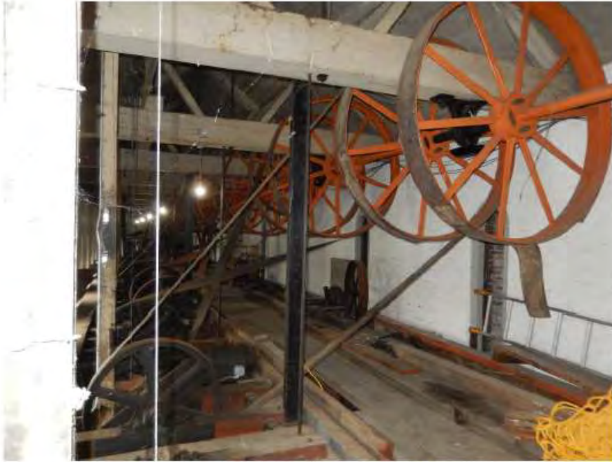
Figure 5-4. Pawtucket Gate House, belt-and-line shaft system.
