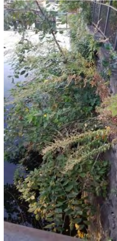
Polygon No.: 51 Photo No.: 51 Date: 9/26/2019 Direction Photo Taken: Northeasterly Description: Vegetation growing on the canal wall include trees, such as mulberry and elms, and herbaceous ragweed.
