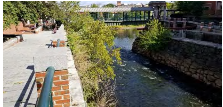
Polygon No.: 7 Photo No.: 7a Date: 9/25/2019 Direction Photo Taken: Easterly Description: Several large woody trees including river birch, tree of heaven, and silver maple, all approximately 2 to 5 inches diameter at breast height are growing out of the canal wall.
