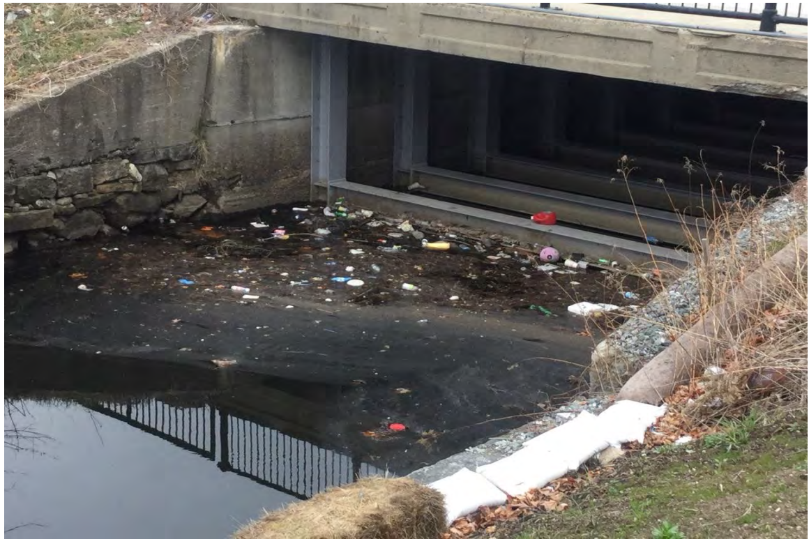
Photo 5-2. Waterborne trash on the Western Canal at Merrimack Street.
