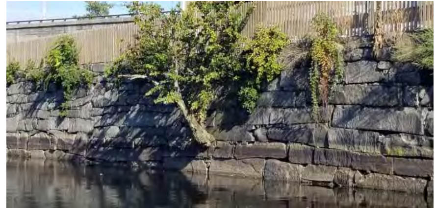
Vegetation Point No.: VP-16 Photo No.: VP-19 Date: 9/26/2019 Direction Photo Taken: Northerly Description: A small clump of mulberry are growing out of the canal wall.
