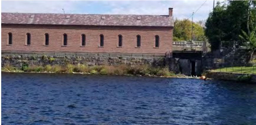
Photo Location No.: P-6 Date: 9/26/2019 Direction Photo Taken: Easterly Description: View of Pawtucket Gatehouse. Vegetation is growing on debris deposited against the gatehouse.
