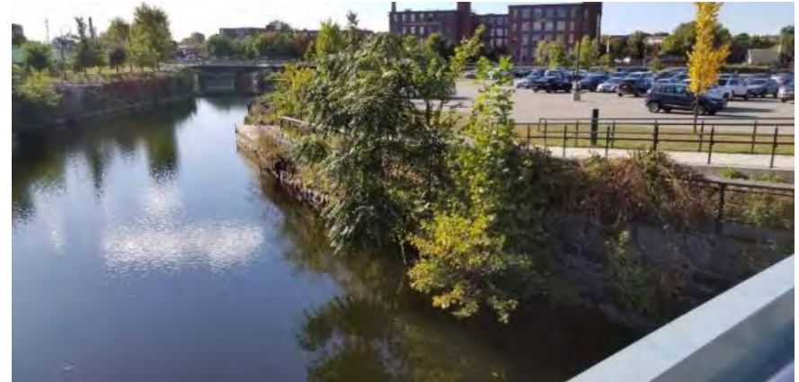
Polygon No.: 25 Photo No.: 25 Date: 9/25/2019 Direction Photo Taken: Northerly Description: The vegetation growing out of the canal wall includes one sycamore, several tree of heaven, glossy buckhorn, and ragweed.
