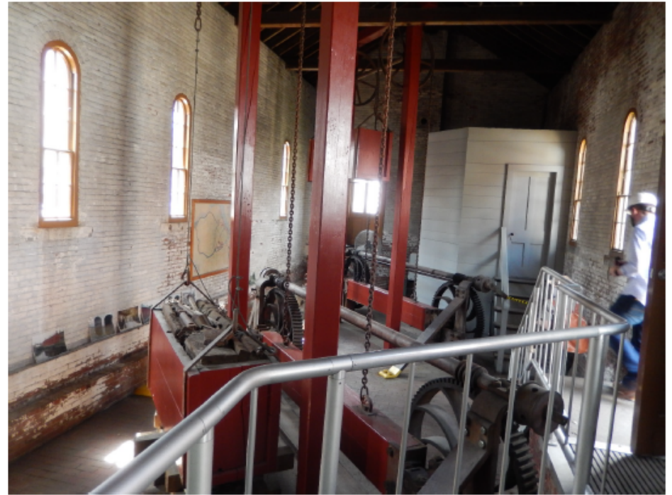
Figure 6-1. Moody Street Gate House, gate hoisting mechanisms.
