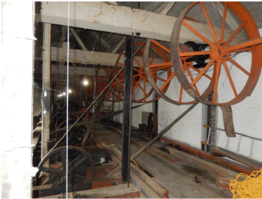
Figure 5-4. Pawtucket Gate House, belt-and-line shaft system.
