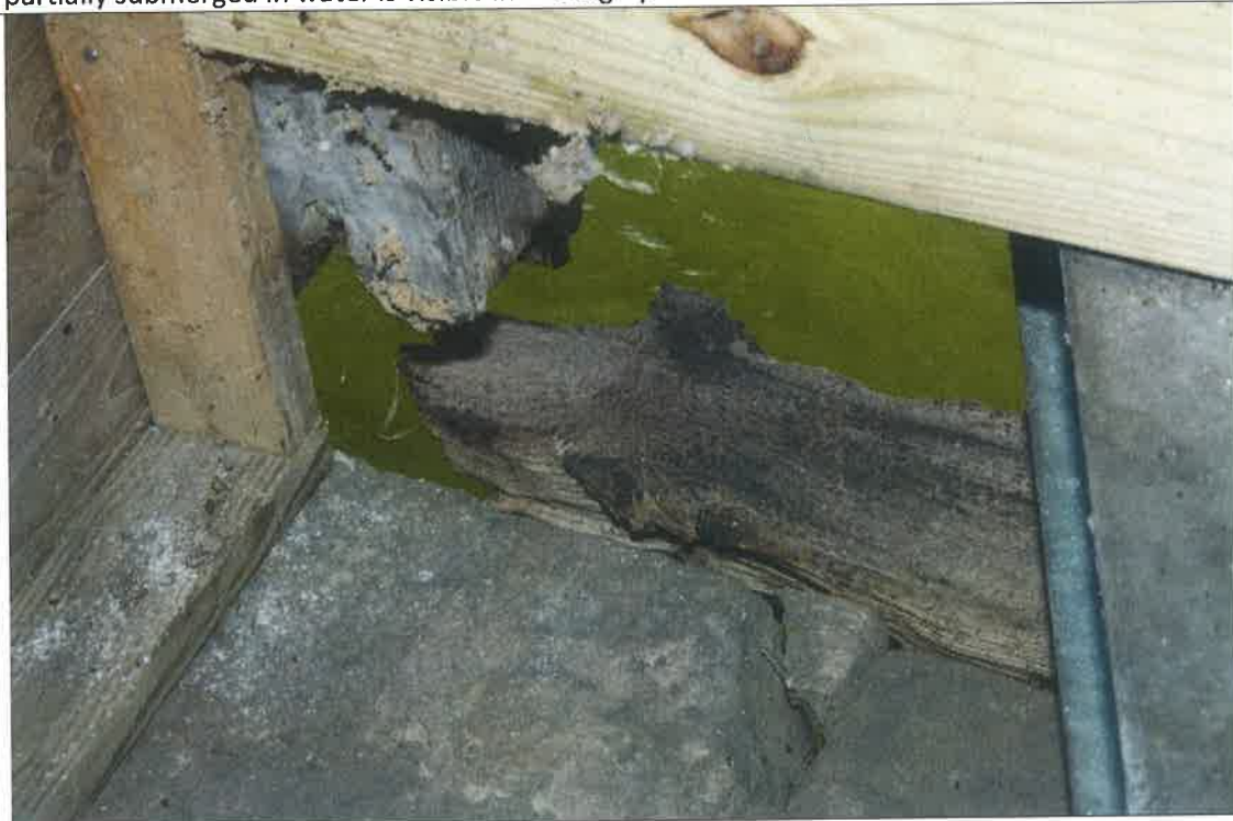
Photograph 8 – Deteriorated heavy timber ledger and wall sill plate at eastern end of south wall.
