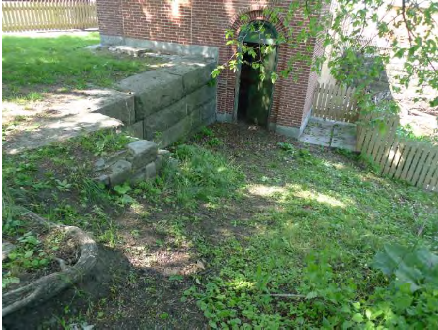
PHOTO 06: LOWER GATEHOUSE DOOR AND WASHED OUT GRANITE STEPS
