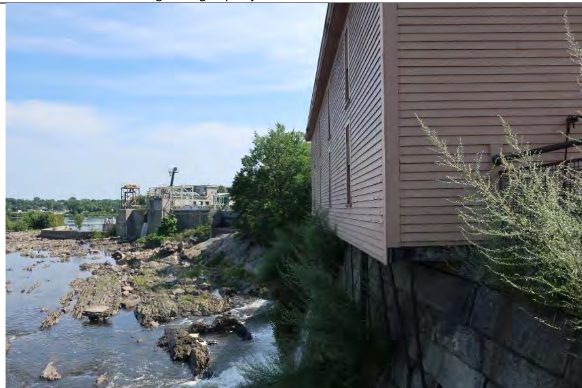
Photograph 10 – North face of dam and gatehouse building; note vegetation growing on face of dam and significant water flowing through dam.
