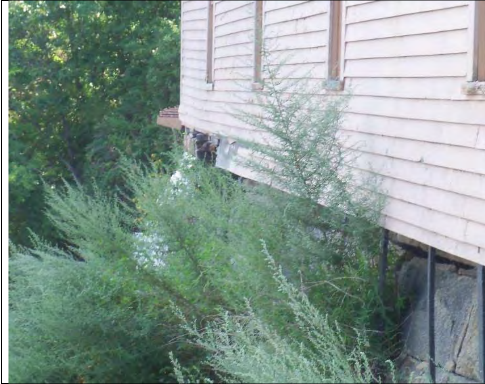
Photograph 3 – Deteriorated / missing sill and missing siding boards at eastern end of north wall; entire building has settled in this area, as evidenced by the downward curvature of the siding boards under the left-most window.
