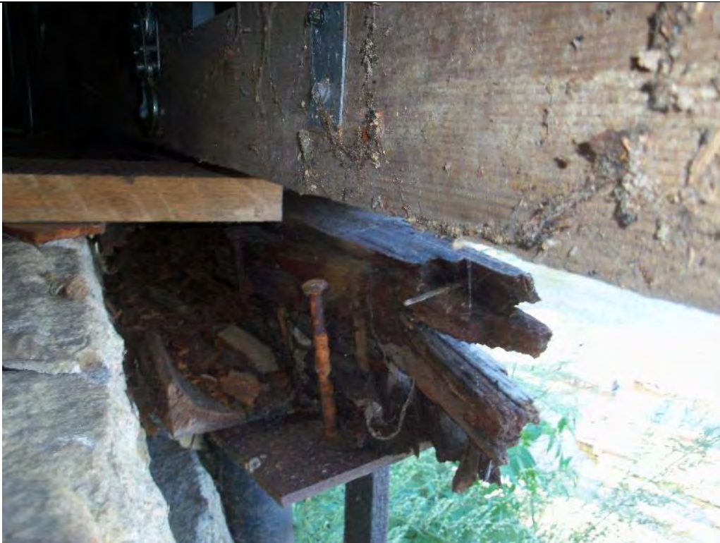
Photograph 4 – Deteriorated / missing sill under eastern edge of north wall; note large gap between dam and wall.
