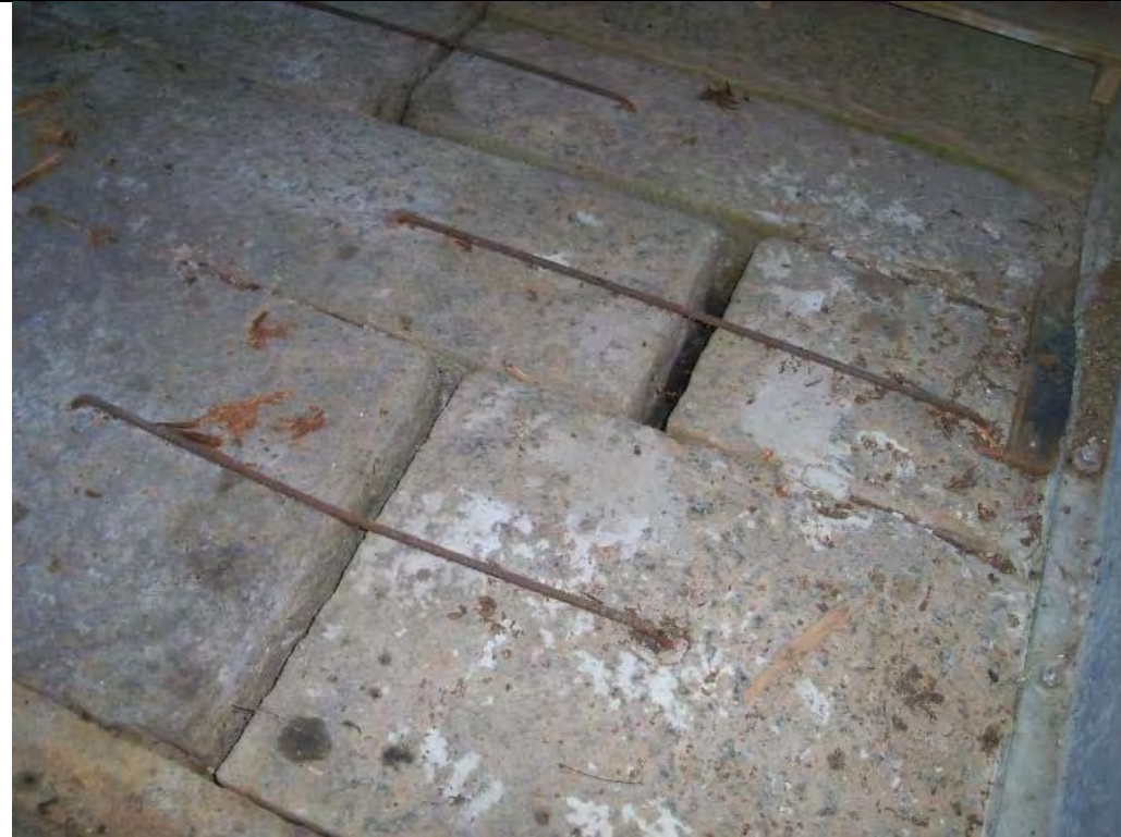
Photograph 9 – Capping stones atop dam, inside gatehouse building; several units have separated, and water can be seen flowing through open joints.
