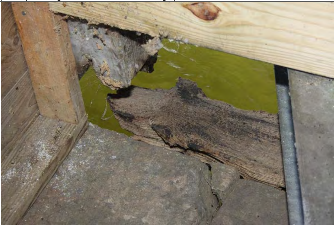
Photograph 8 – Deteriorated heavy timber ledger and wall sill plate at eastern end of south wall.
