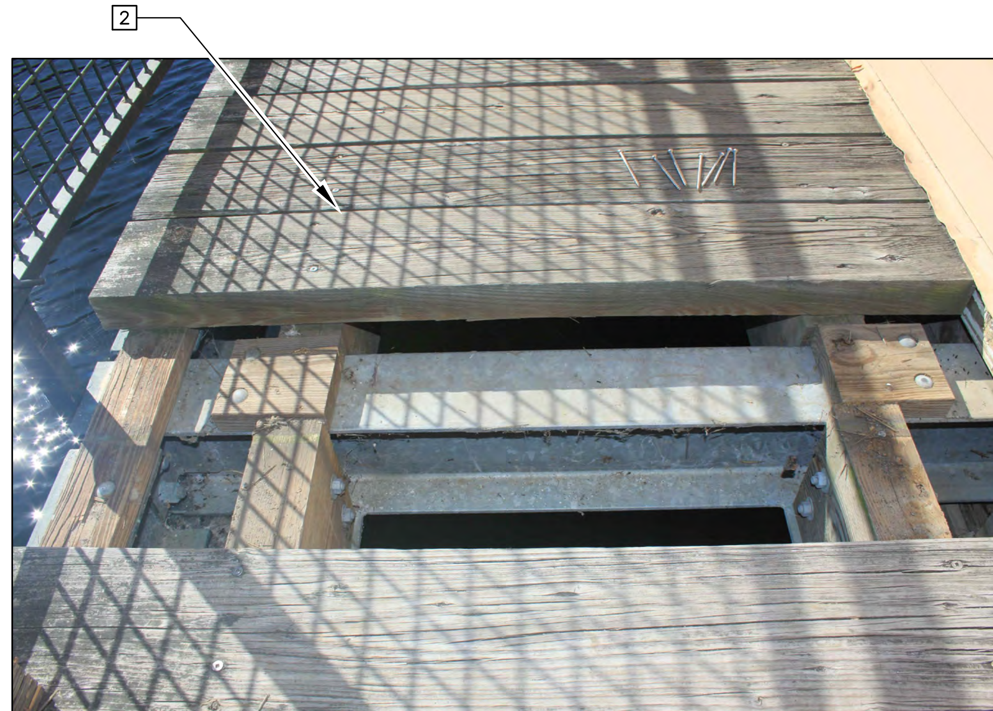
8 PHOTO 8 @ WALKWAY WITH DECKING REMOVED A5
