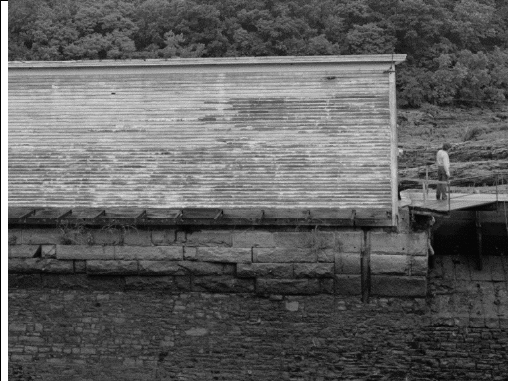
Photograph 5 – HAER Photograph MA-8C-2, taken in 1974 or 1975; note staining in wall and vegetation in joints below gatehouse, indicating that the normal elevation of the Northern Canal was several feet below what it is today. Also, note many open joints in larger masonry units at the top of the dam.
