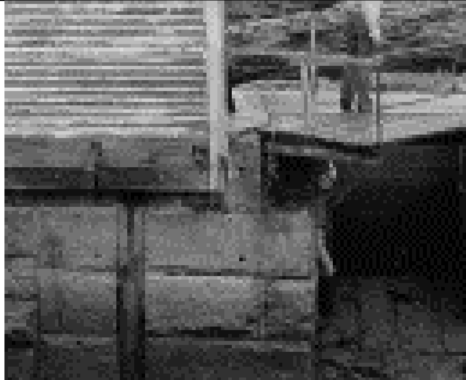
Photograph 6 – Close-up of HAER Photograph MA-8C-2, taken from Photograph 5, showing heavy timber ledger and wall sill.
