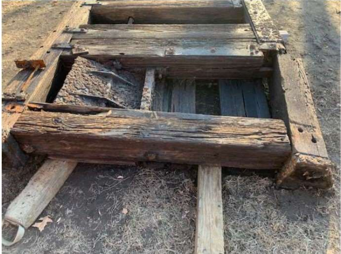
Photo 5-4. Photo of wear of submerged portion of the Northern Canal Gate removed for repair.
