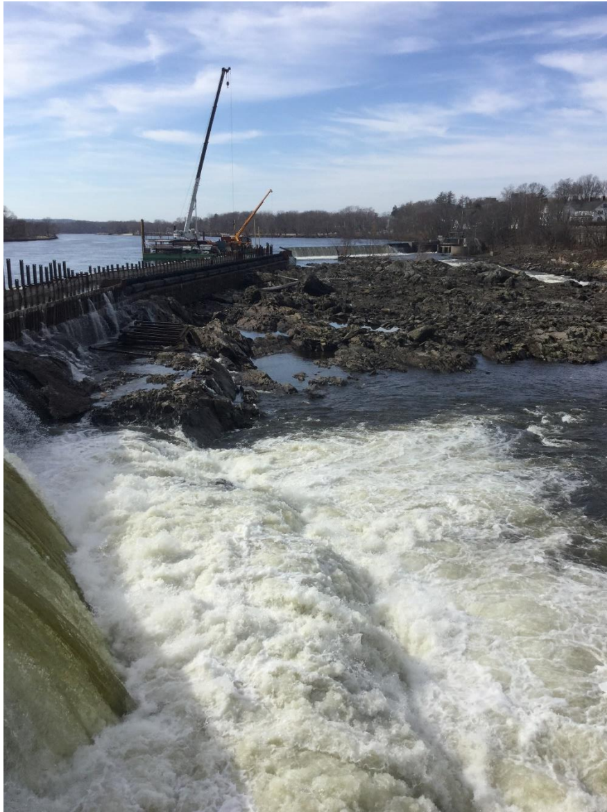
Figure 5.9-4. Pawtucket Dam from Pawtucket Gatehouse (pneumatic crest gate system currently being installed).
