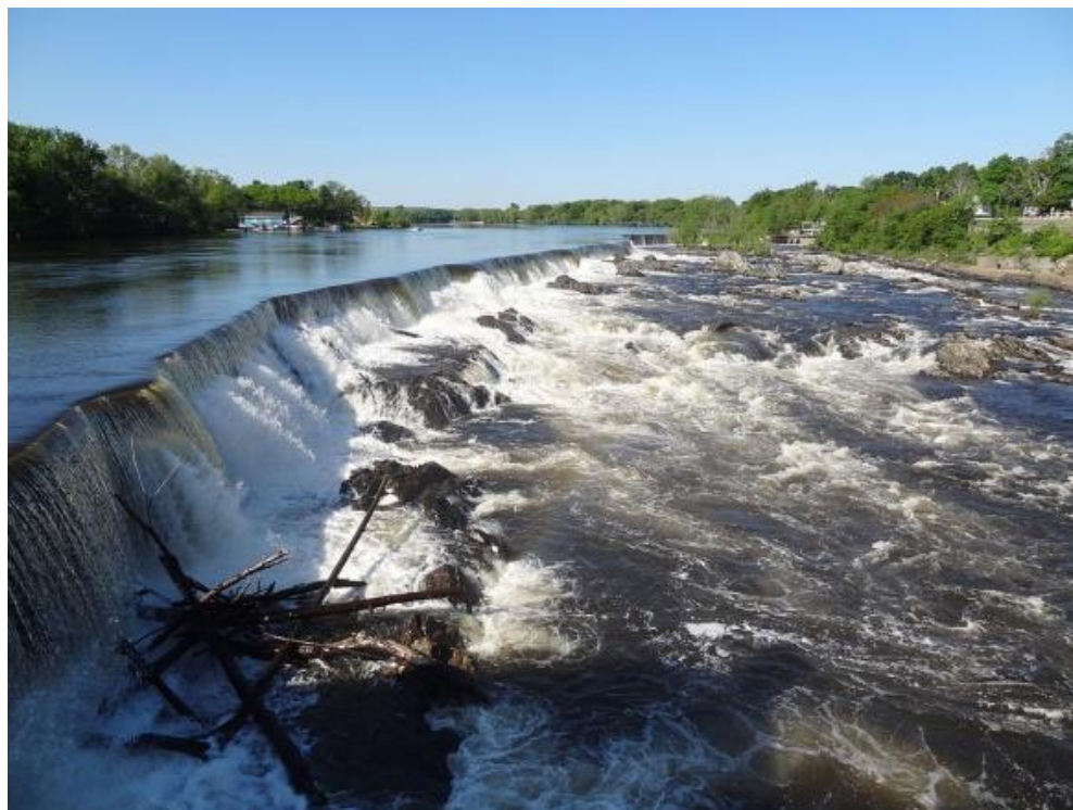
Figure 4.1-1. Pawtucket Dam (prior to the installation of the pneumatic crest gate system).
