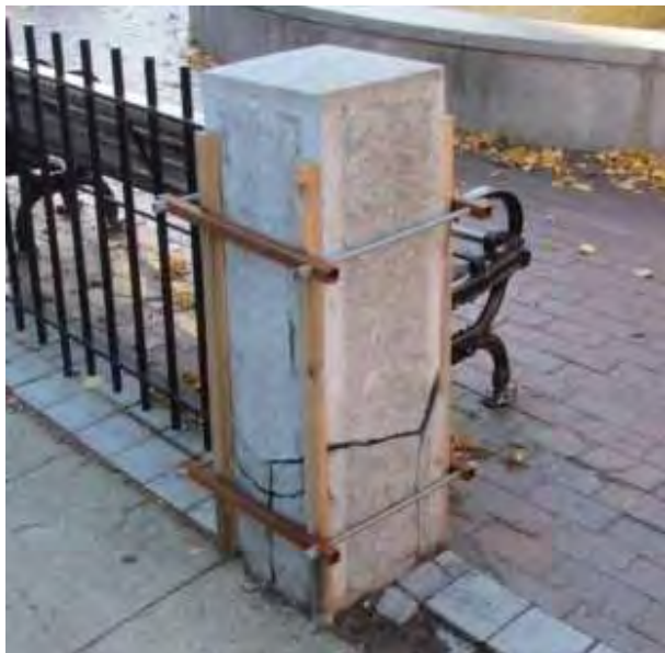
A cracked granite post and temporary wooden support structure in the Mack plaza. (DCR)
