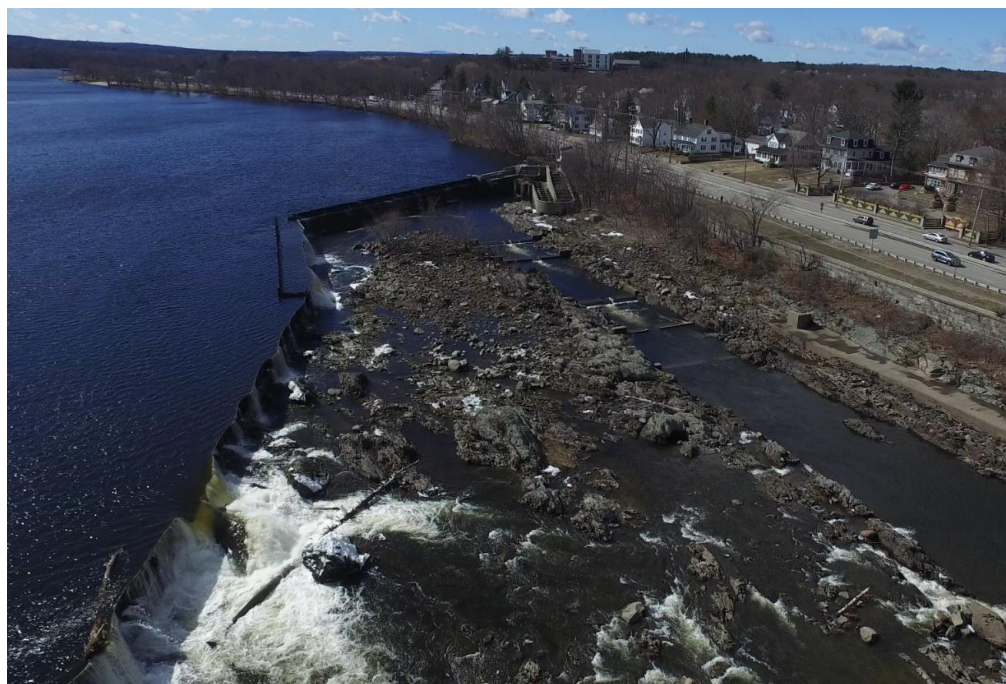
Figure 4.1-2. Pawtucket Dam and concrete fish ladder with partially installed pneumatic crest gate system adjacent to the fish ladder.
