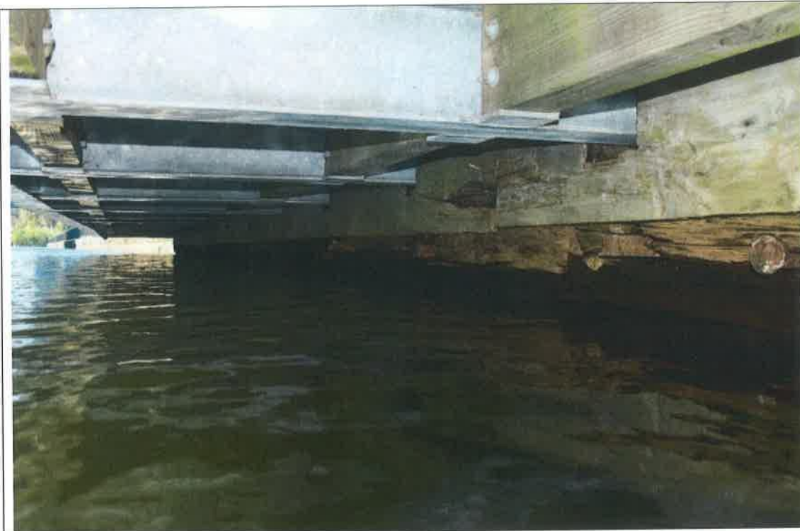
Photograph 7 – Underside of walkway along south side of gatehouse; the deteriorated sill that is now partially submerged in water is visible in Photographs 5 and 6.
