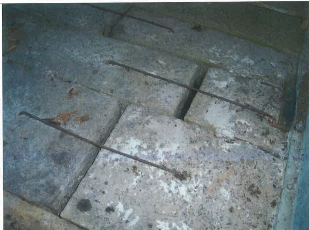
Photograph 9 – Capping stones atop dam, inside gatehouse building; several units have separated, and water can be seen flowing through open joints.
